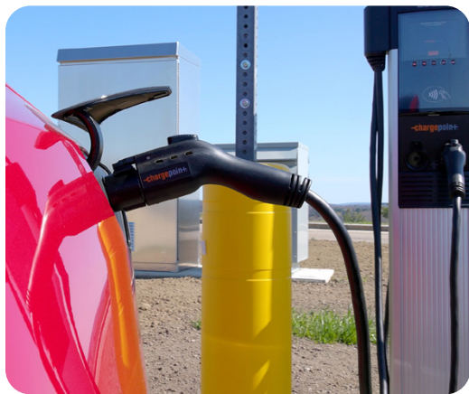
New EV charging stations at Main Parking lot
