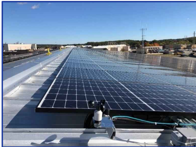
Figure 11-8 Boston MedFlight's 200 kW Rooftop Solar PV Installation
