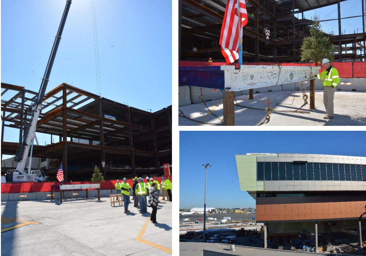
Terminal E Renovation and Enhancements Project under construction (left, top right). Completed project section (bottom right). Source: Massport
