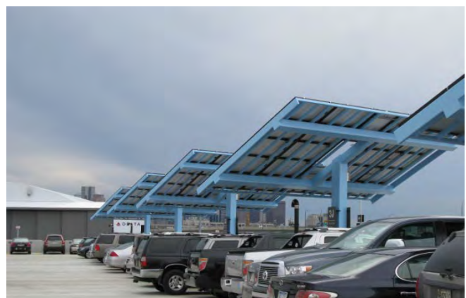
Solar panels at on the roof of the new Logan Airport Parking Deck (Economy Parking).
